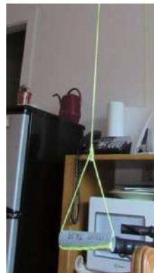
Emergency pull cord
